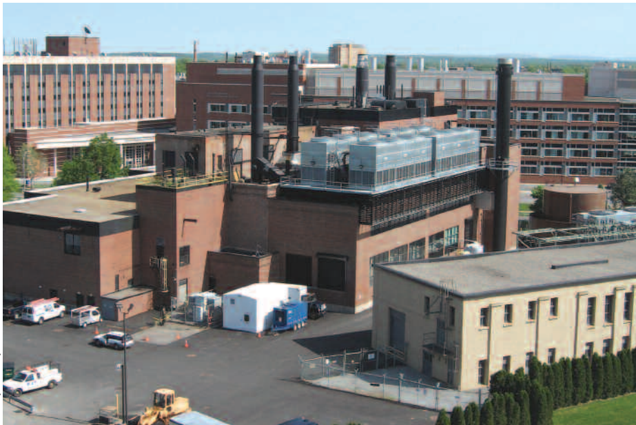
The University of Rochester's new cogeneration facility can produce up to 250 MMBtu/hr of hot water for the hot water district heating system and 25 MW of electricity. Although cogeneration had been a topic of discussion at the University of Rochester since institution's early days, the technology was finally implemented with the startup of this new plant in 2005.
